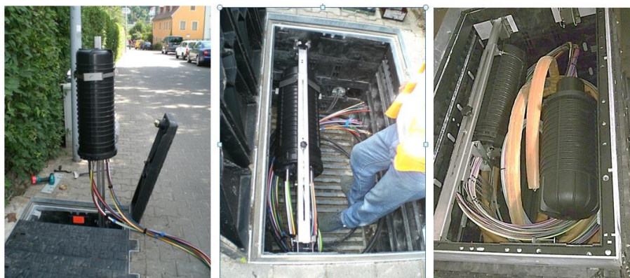
Figure 13: Underground fibre distribution with closures
