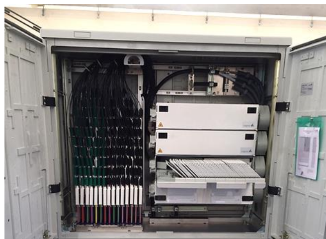
Figure 14: FTTx fibre distribution cabinets often have limited space available
